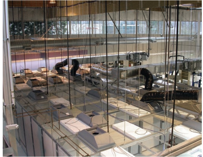
Ceiling-mounted HVAC equipment serving the production area.
