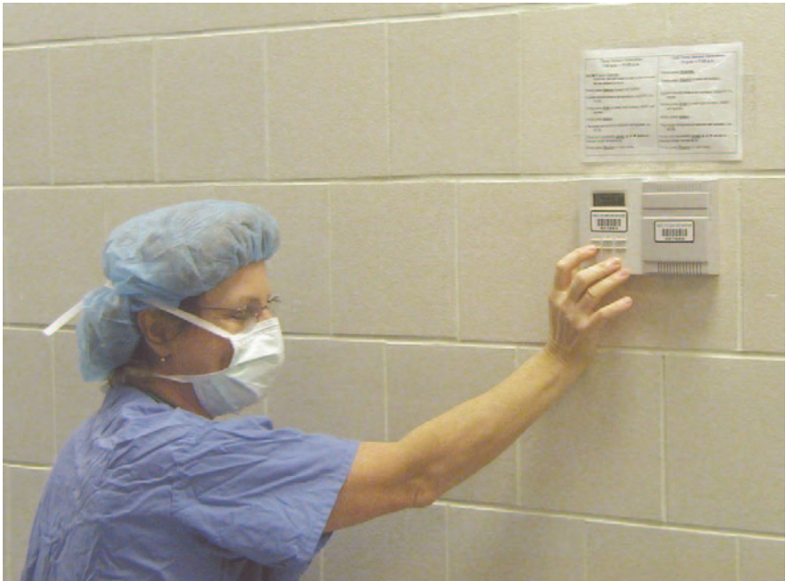
Mounted on the wall in each OR is an intuitive, six-button sensor with LCD display. The sensor allows the medical staff to adjust the room's temperature and can override the hospital's night setback mode in preparation for an emergency after-hours surgery.
